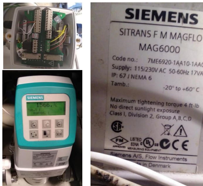
Fig. 29. Siemens water flow meter and transmitter.
